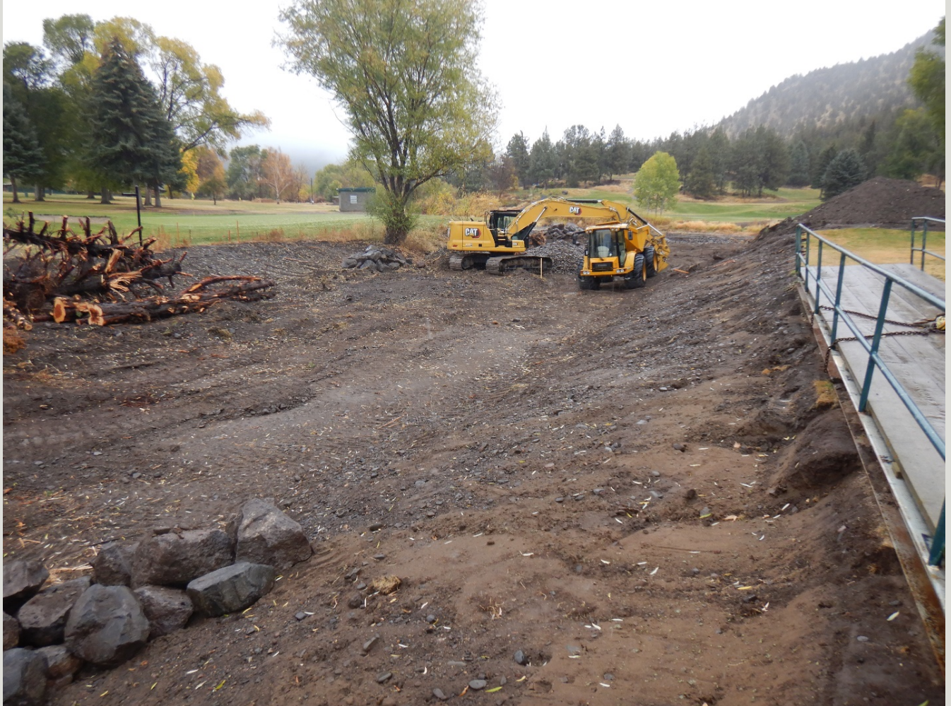
Key instream structures being placed and buried (anchored) in Ochoco Creek - October 2022
