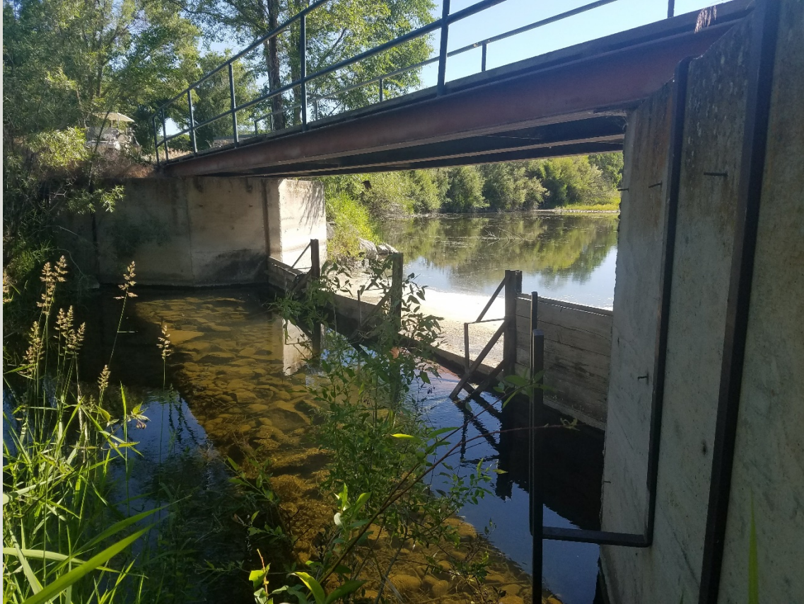
Existing diversion structure with flashboard configuration for managing pond water levels (pre-project)
